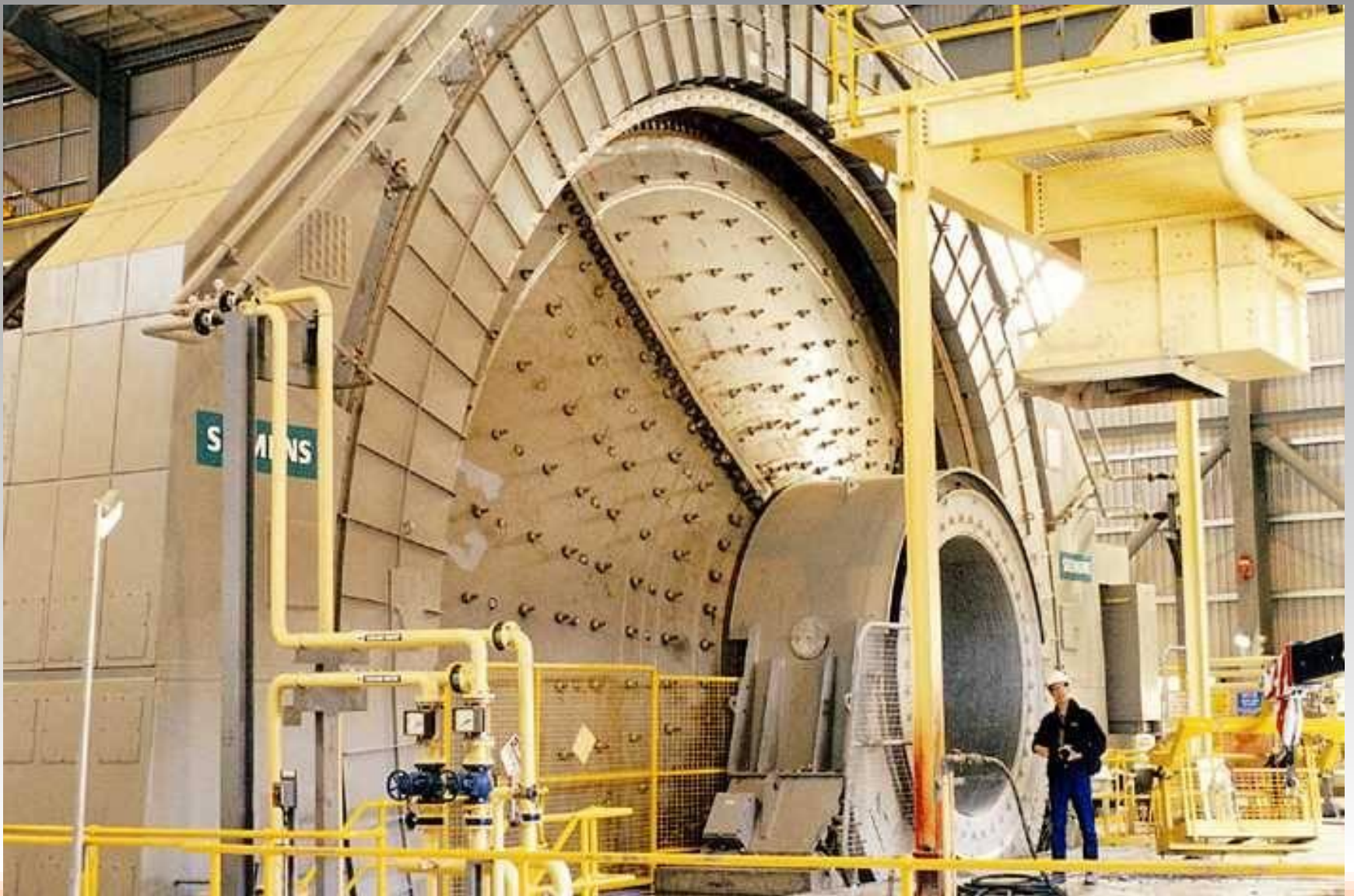
Newcrest Cadia SAG mill, 40', 20 MW
