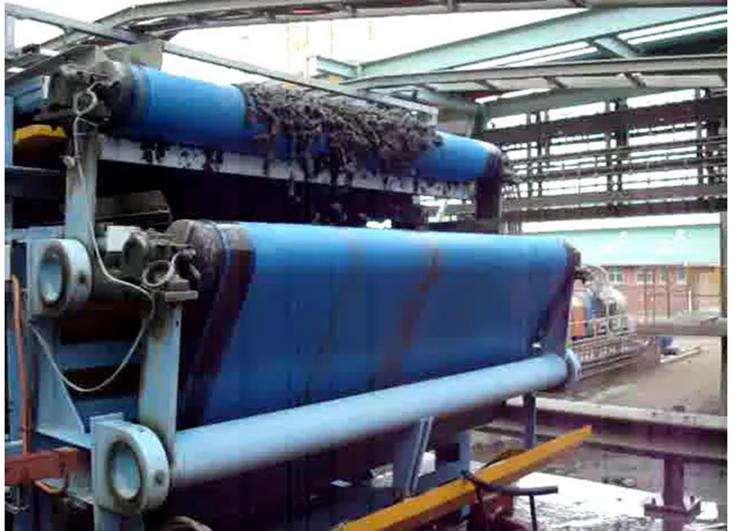
Belt Press Dewatering
