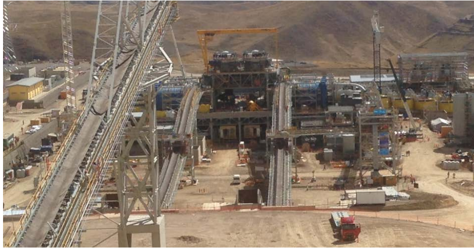
Figure 7 - Constancia grinding circuit viewed from the primary crusher
