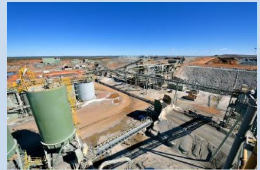
The crushing and grinding circuit at Sunrise Dam
