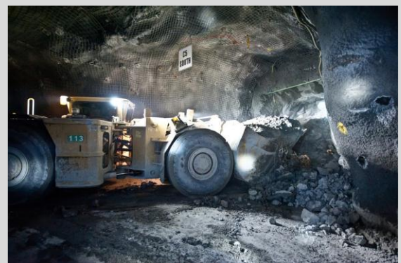
A scoop mucks out an underground draw bell. Overhead rock collapses into the draw bells to be extracted.
