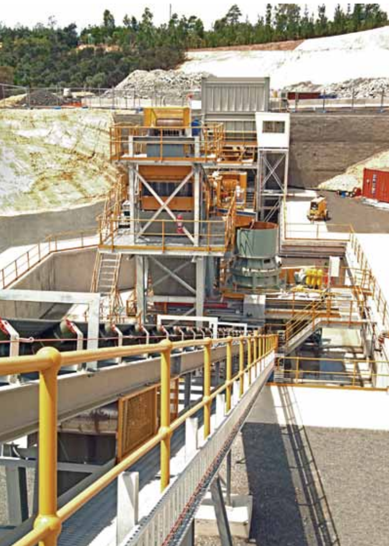
The Castlemaine Goldfields Ltd Ballarat gold project has a three-stage crushing only comminution circuit minimising comminution energy consumption
