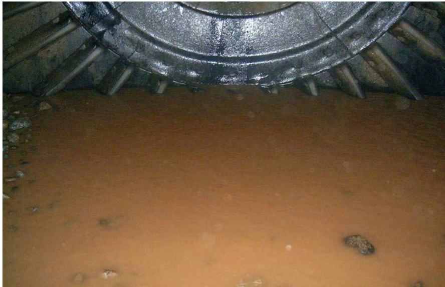
Figure 2 - Crash stop of SAG mill showing pooling
